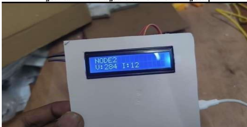
Fig 4: LCD-Based Monitoring Output of Voltage (284 V) and Current (12 Amp)
