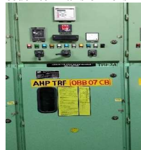
Fig 9 OUTGOING TO TRANSFORMER
