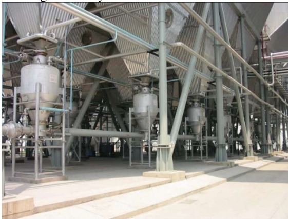
Fig: 4 Ash handling plant
