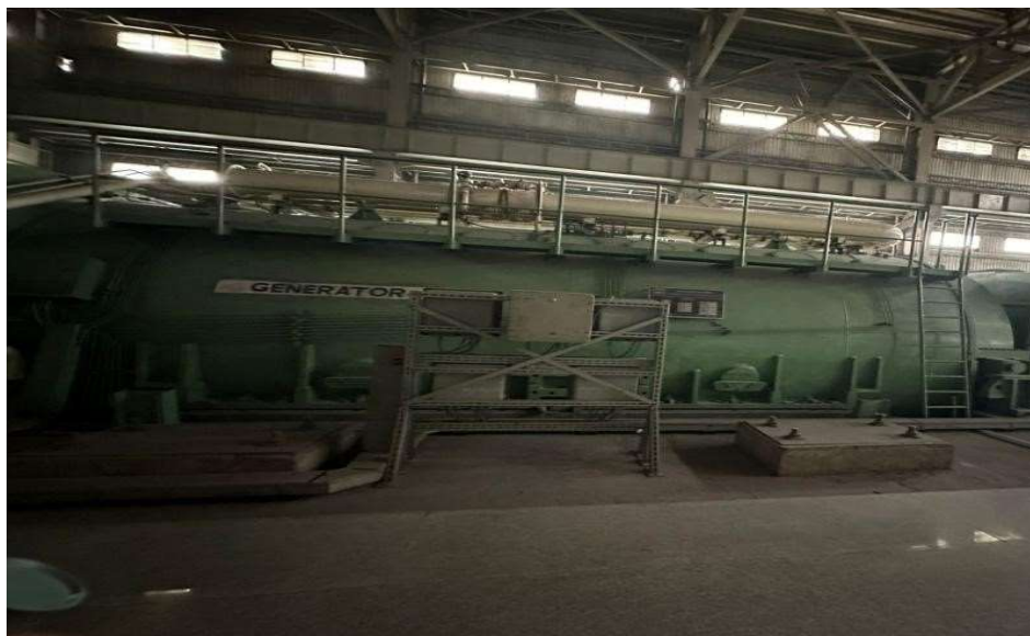
Fig 3.1 Generator at KTPS
