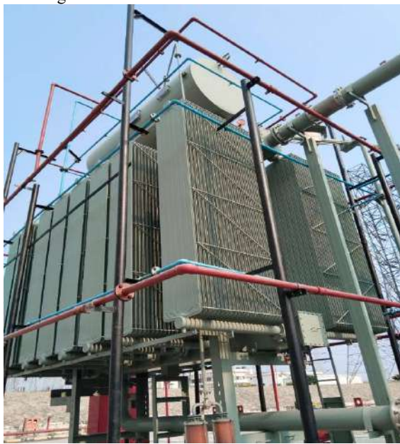
FIG:5.7: REACTOR IN 400KV
