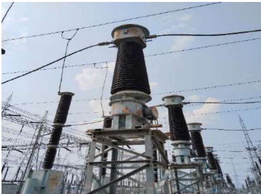
FIG:4.6: CURRENT TRANSFORMER
